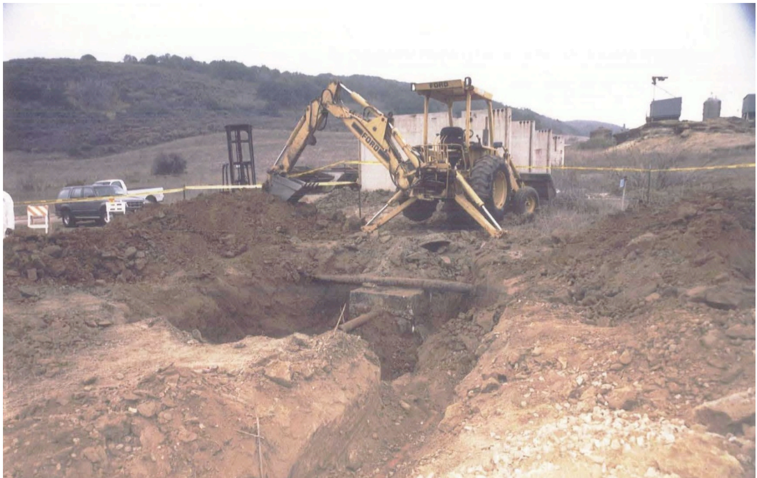
The above photo may help in some identification of pipes to and from Building 4011, this is the 2001 excavation of the Building 11 Leach Field.
