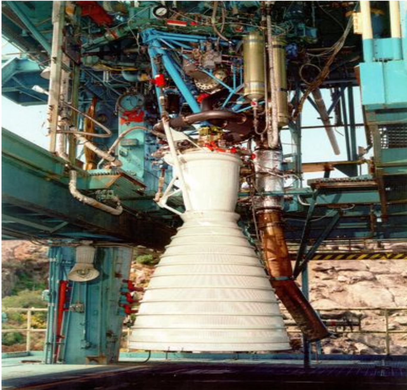
RS-27A Engine Installed in Alfa Test Stand Santa Susana Field Laboratory (SSFL) - 1999
