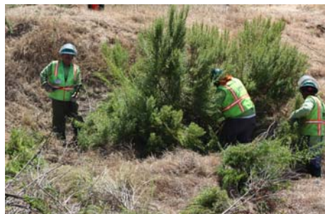
Vegetation clearing performed in sections of Area IV at SSFL to allow for proper operation of gamma scanning equipment.
