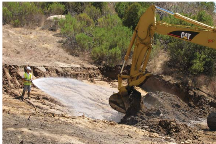
Water was used as a dust control measure when soil was removed from the outfall and loaded into transportation truck
