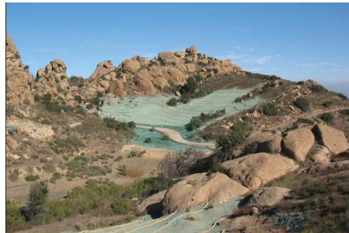
After soil was removed, excavated areas were back filled, recontoured and hydroseeded.
