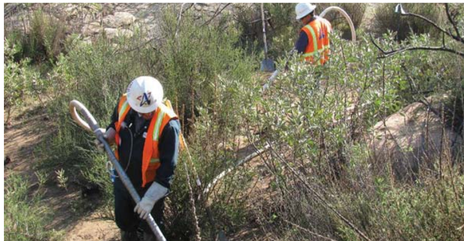
Workers use hand vacuums to remove lead shot from the rock outcrops on Sage Ranch.
