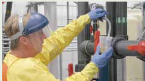
Groundwater Extraction Treatment System – Groundwater from an extraction well is pumped through the new treatment system using a series of regulatory-approved technologies to remove chemicals.
