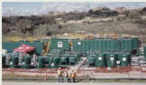
Storm Water Chemical Treatment System – During the rainy season, in order to meet our stringent permit limits, we collected storm water runoff in holding tanks and treated it with advanced filters and chemicals before release. (Image courtesy of Simi Valley Acorn)
